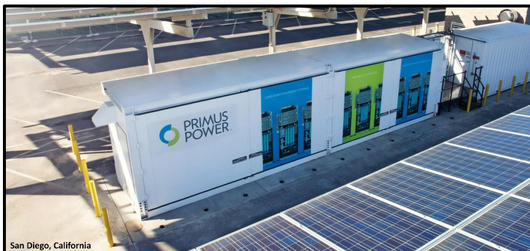
Figure 3. A high-resilience microgrid implemented at the Marine Corps Air Station at Miramar that employs a Primus Power 1 MWh battery system to firm solar power.
